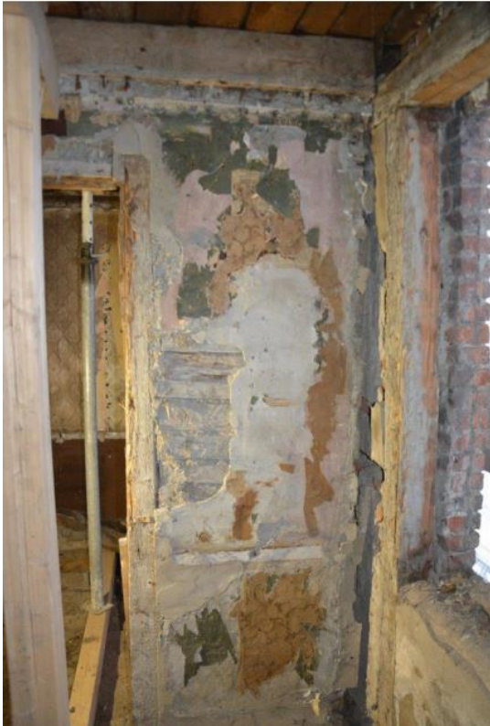
03 Traditional type of vernacular Nordic timber and earthen construction (earth mortar layer between squared timber in wood framing) with “rapping” (a type of Norwegian clay plaster on wooden surfaces), in the house Smedbakken 5 from 1845/46 in Trondheim, Norway (source: author)
