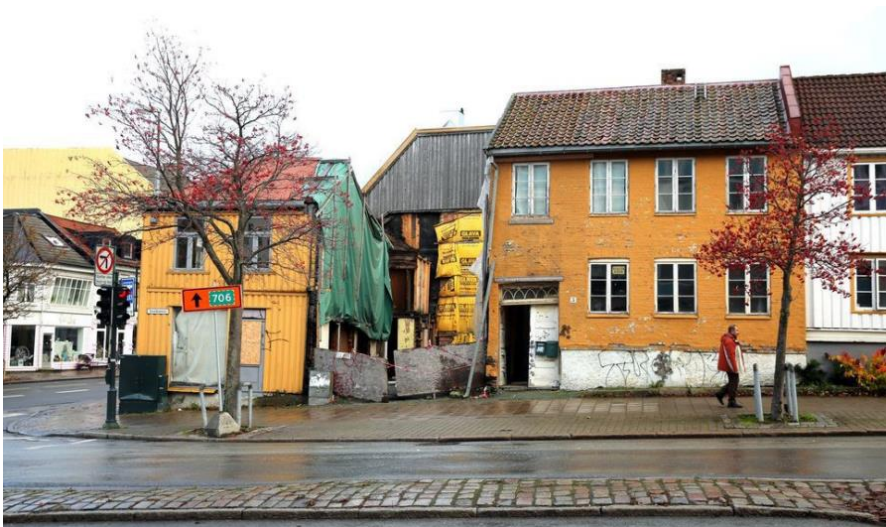
01 The façade of Smedbakken 5 in Trondheim built in 1846: approx. 40-year-old paint that acts as a vapour barrier and visible damage to the building physics caused by disturbed micro-meteorology: frost wedging, cracks and flaking of the paint (source: Adresseavisen)
