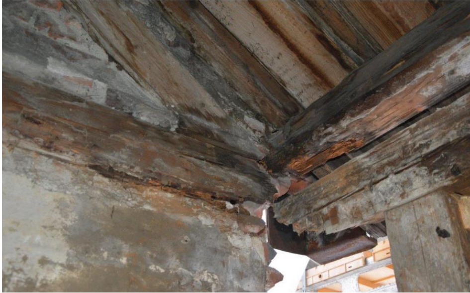
02 All of the geometric envelopes of the 175-year-old residential house are affected due to the micro-meteorological reversal of the vapour permeability and the following change of the dew point. (Source: Author)
